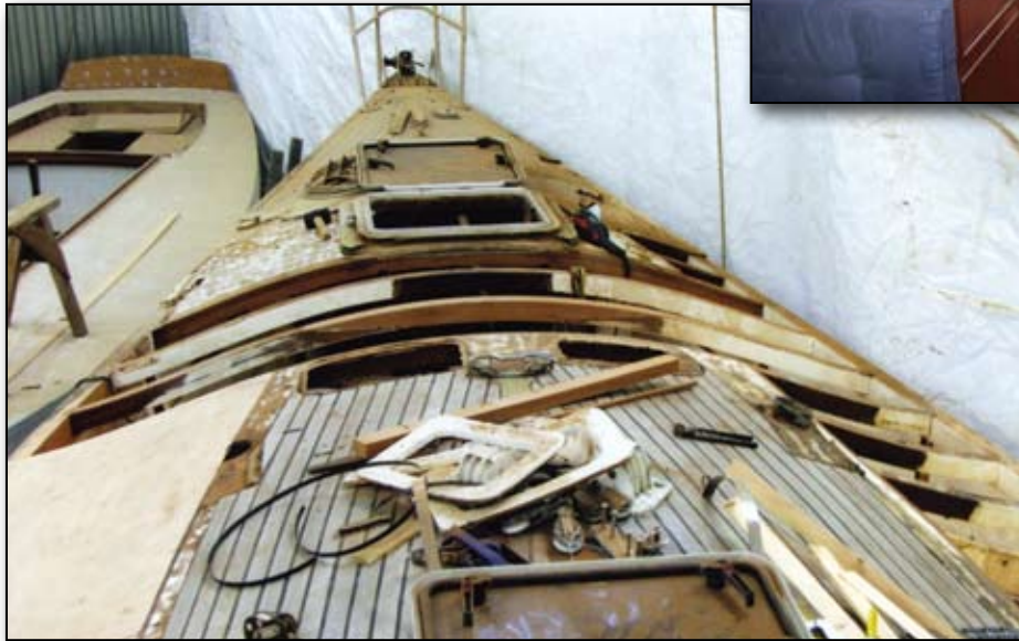
Her restoration was a labour of love as much rotted timber had to be replaced.
